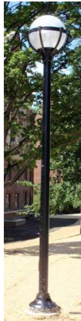
typical pedestrian scale light pole
